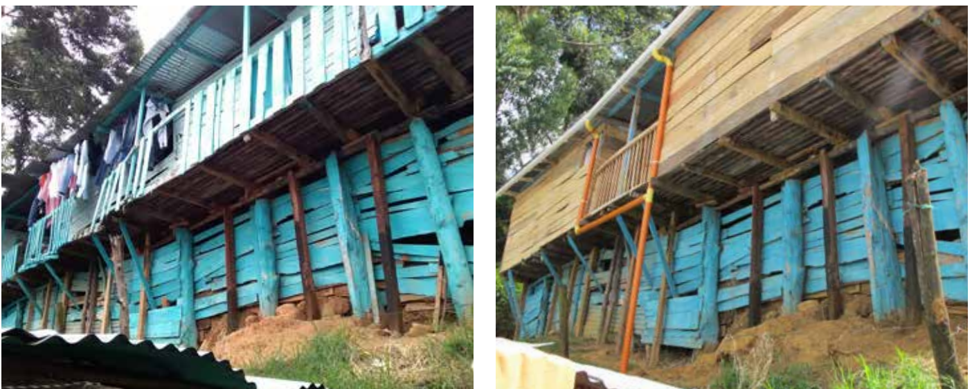
Figures 14 and 15: This is the house of a resident called “La Mona” (monitoring point number 2) showing before (left) and after (right) the mitigation works. Source: Research Team.
