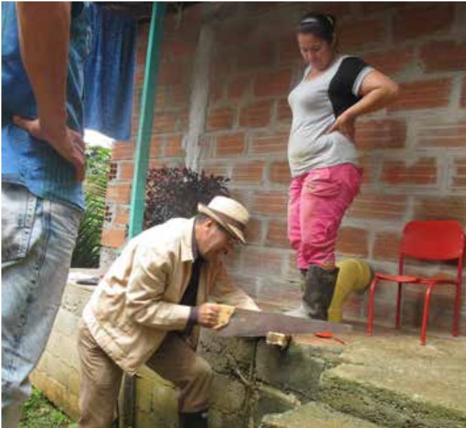
Figure 12: The research team consisted of professionals with technical knowledge of construction techniques that was made available to the residents. Here one of the team members shows a resident how to prepare timber shuttering prior to pouring the concrete. Source: Research Team.
